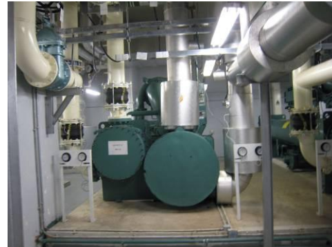
Photo 15: Eleven sets of chiller are installed.
