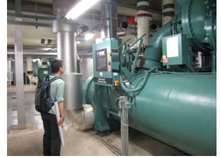
Photo 13: Centrifugal-type water-cooled chillers.
