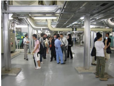
Photo 14: Central chiller plant.
