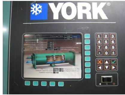
Photo 12: The operating parameters of the chiller can be programmed to suit different requirements at night time and during weekends and holidays.
