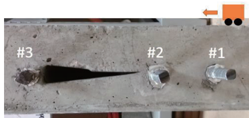
Figure 4: Design of specimen D2. An artificial air gap in wedge shape is situated between rebar #2 and #3.
