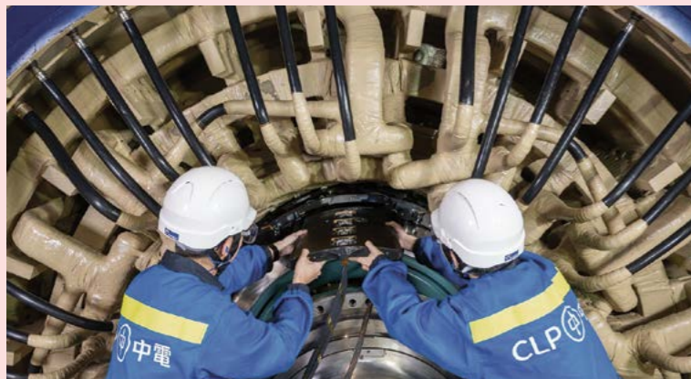
The slim robot is equipped with designs and mechanisms that enable it to 'crawl over' the baffles and complete the inspection automatically.
