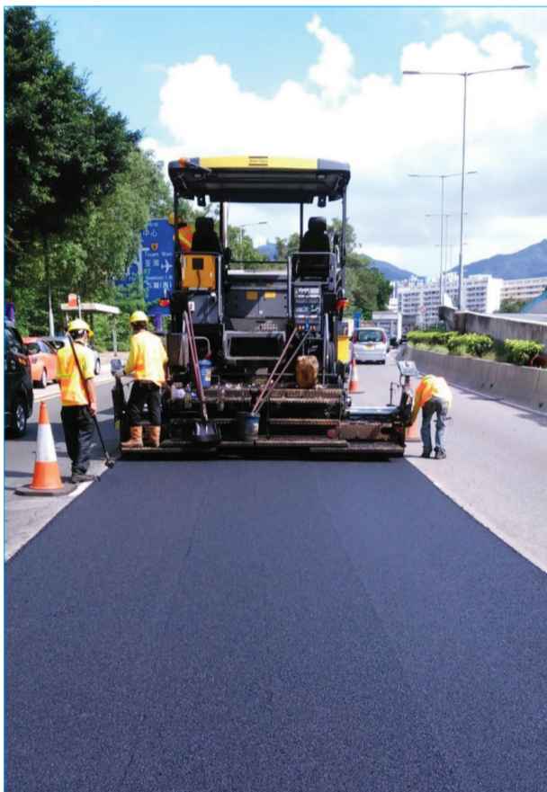
溫拌添加劑能降低施工所需的溫度，減少鋪設路面的能源消耗和排放 The warm mixing additive can reduce the temperature required, thus lowering energy consumption and emission during the paving process
