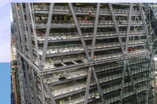
B2 Application of high performance steel materials Q690 to Q960 in super high-rise commercial buildings
