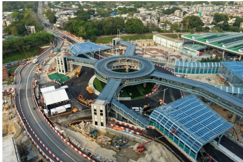
S960 pedestrian overpass at Lung Yeuk Tau Intersection in the Northern Metropolitan Area
