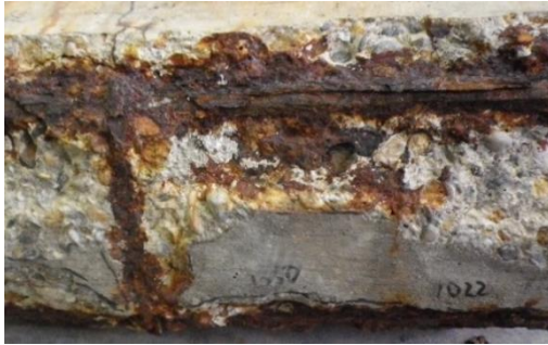
Fig. 2 Image of corroded reinforcement
