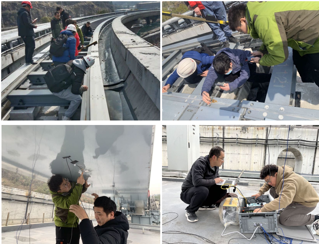
Fig. 2.20 Installation of sensors and monitoring of Fenghuang maglev system
