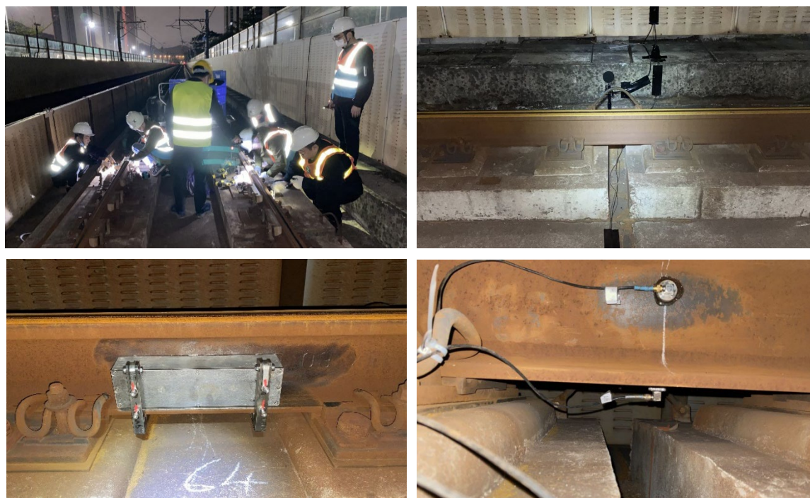
Fig. 2.4 Installation and testing of MRPD in the viaduct line near Tanglang City East station of Shenzhen Metro Line 5
