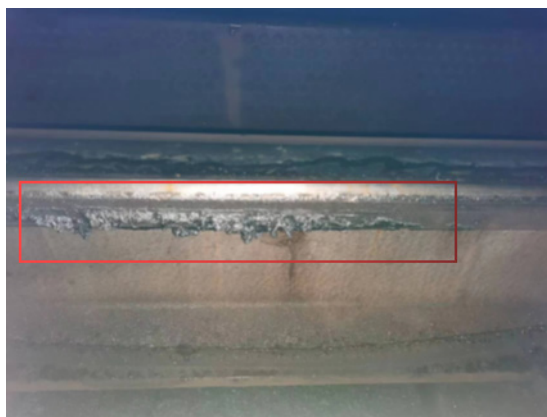
Fig. 2.3 Signs of orbital side grinding and debris
