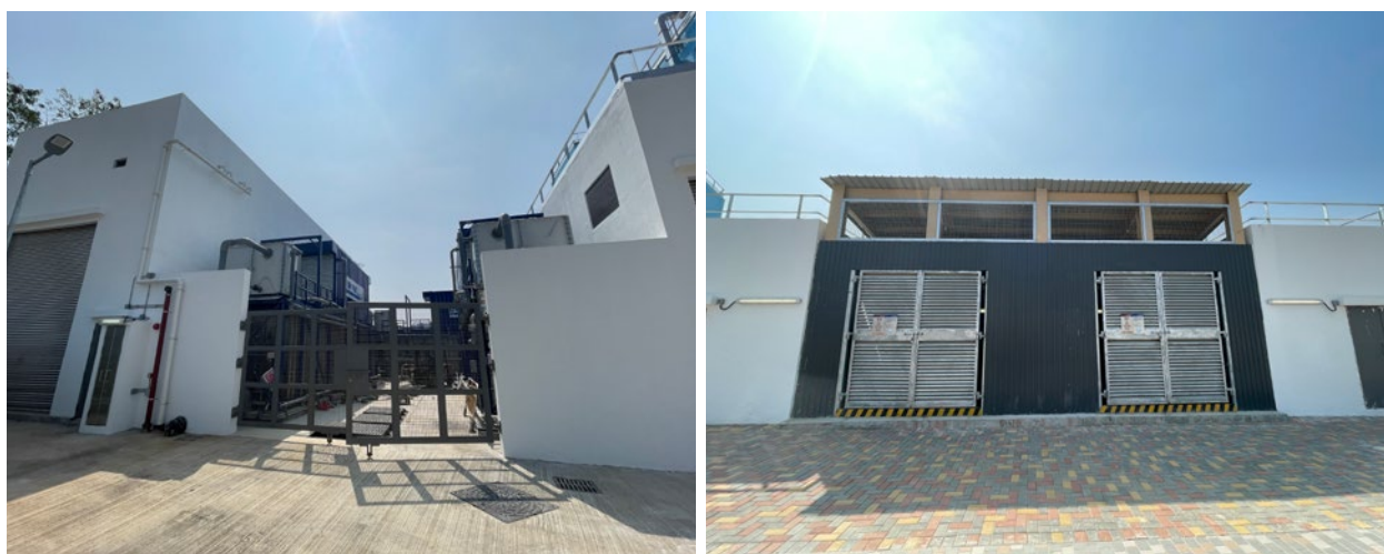
Additional infrastructure including a sewage treatment plant and Electrical & Mechanical plant rooms 額外加設的基建包括污水處理及電機機房
